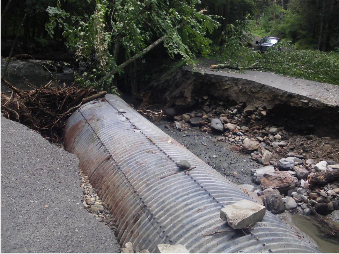
Piggery Road culvert washout – July 29, 2021
