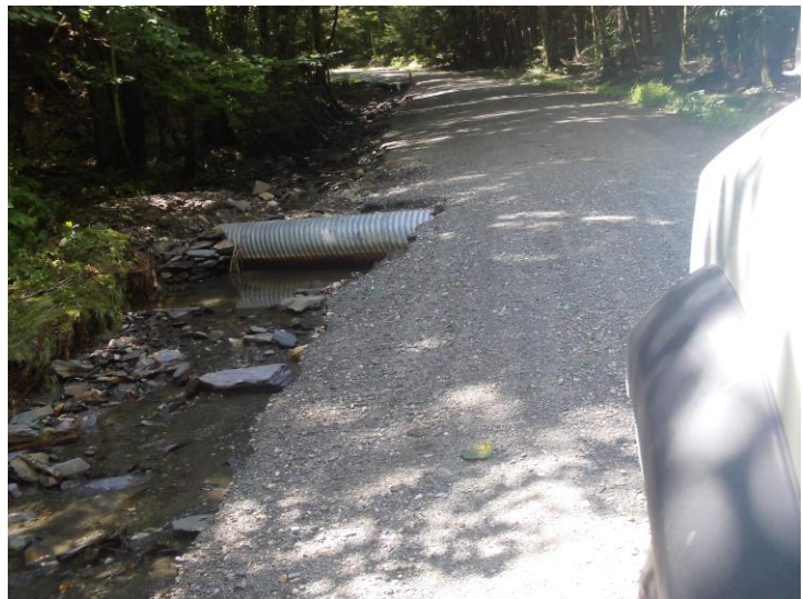
Bemis Road after the July 29, 2021 Storm. – Photo from Town Manager Russ Hodgkins.
